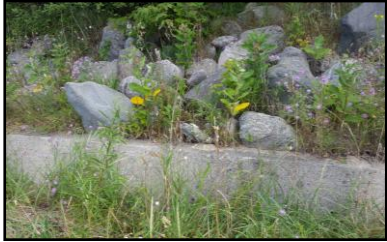
Critical Dune sea wall – Photo BY: TNN
