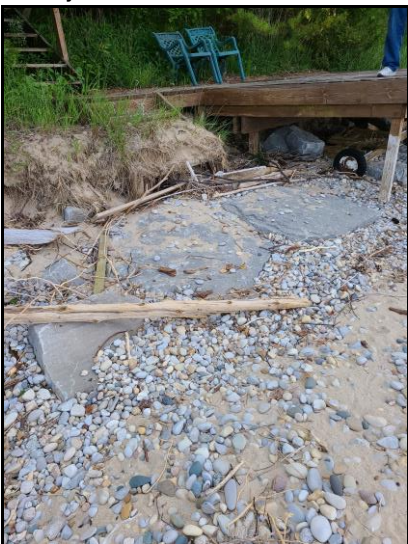
Bluff Toe Protection. Photo By TNN
