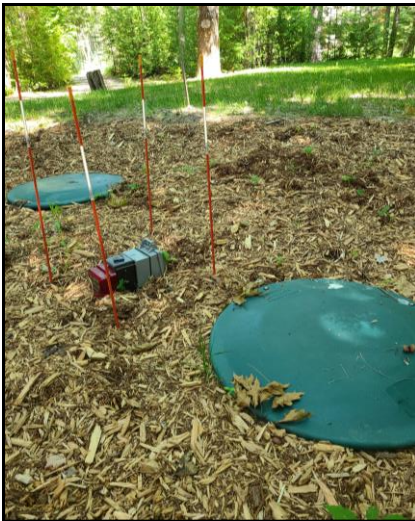
New system cost nearly 2X gravity system plus landscaping. Photo by TNN
